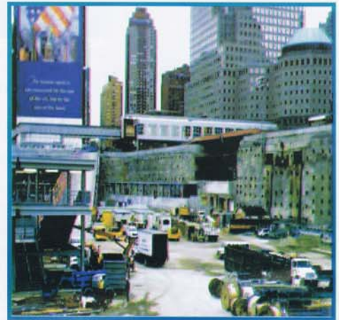
REBUILDING AT WTC SITE The new temporary PATH terminal is now serving over 50,000 riders every day.
